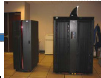
Municipal Court Data Center
